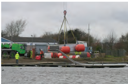
Hydroplates being installed at Kings Mill Hospital, Mansfield (reproduced courtesy of Geothermal International)
