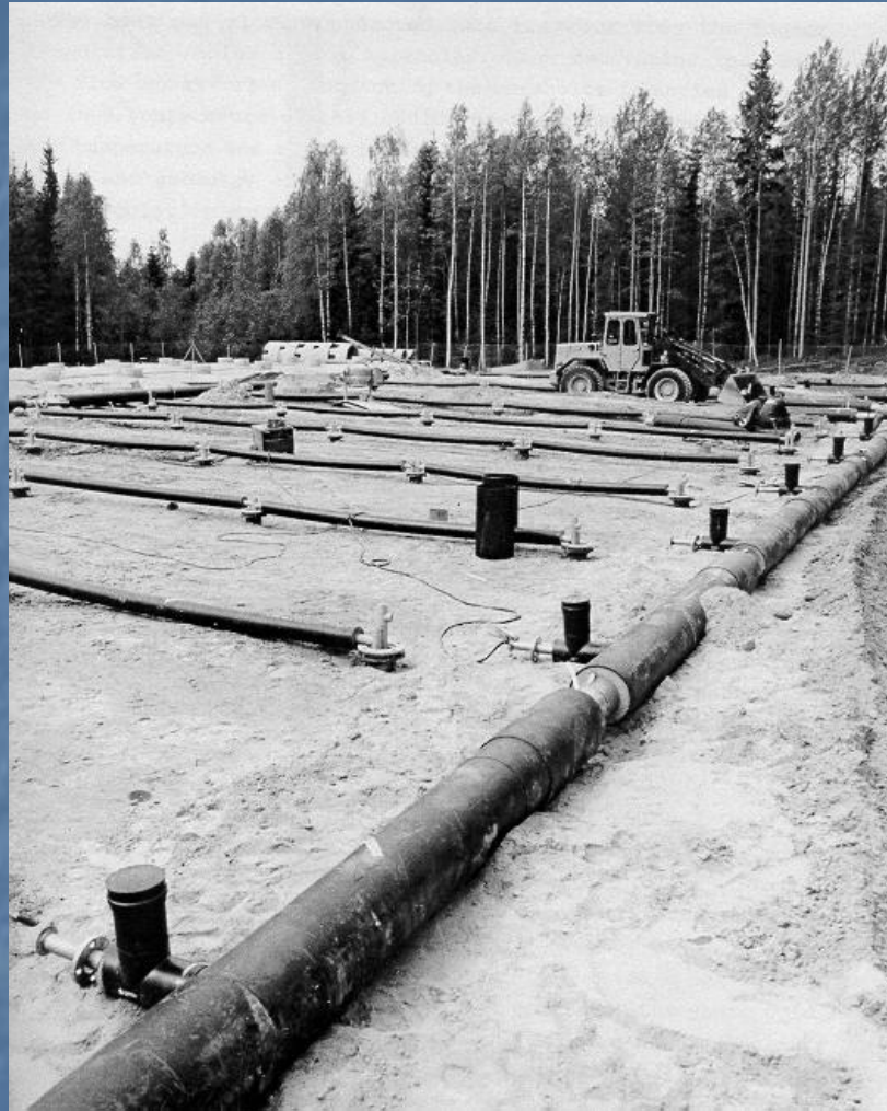
Connection pipes and manifold
