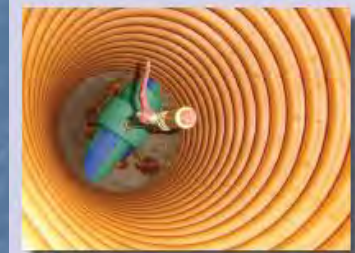
Field manifolds have degassing valves
